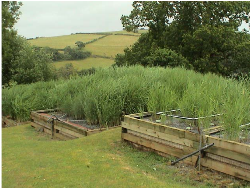
Plate 2 – Timber framed reedbeds at a Milk Processing Plant
